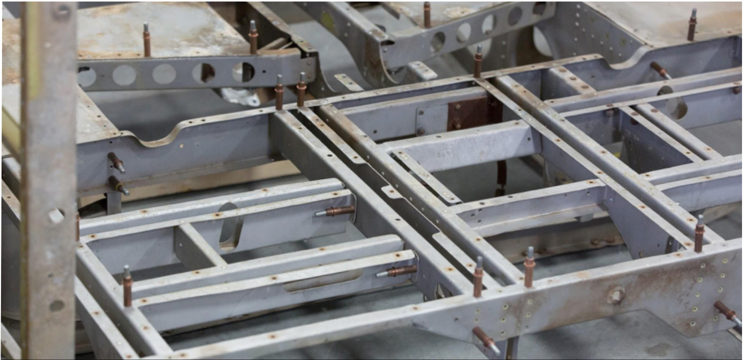
The view here shows floor as it is clecoed together while trial fitting.
