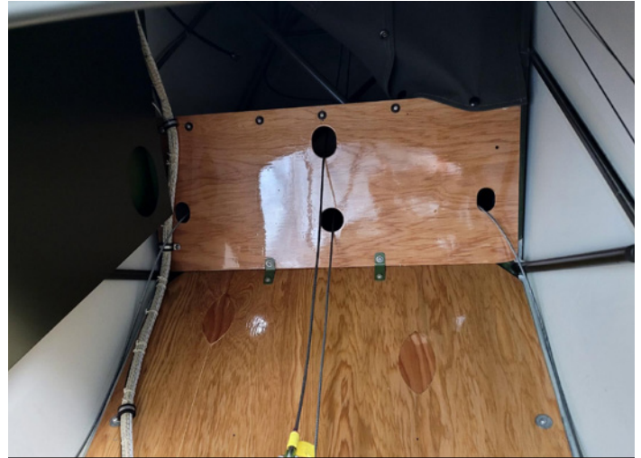
The elevator control cables run back through holes in the plywood lower rear wall of the cabin.
